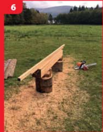
6 Four sides done. Beam has been turned and running rail fixed to flat side of beam.
